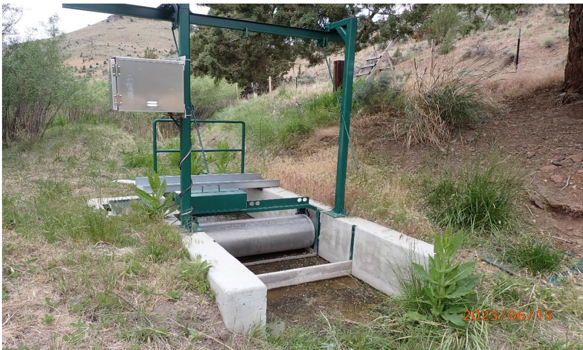
Below: Fish screen and flow measuring device.
