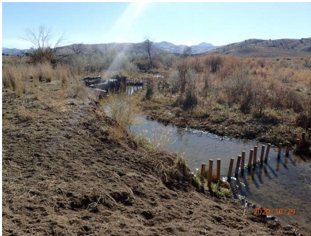
Above: Photo Point #26- Landscape view of BDA structures and large woody debris.
