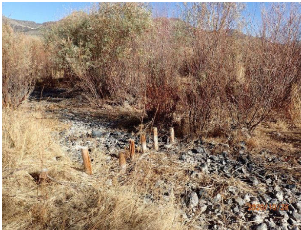
Above: Photo Point #14- Close up of BDA structure with riparian plant species thriving.
