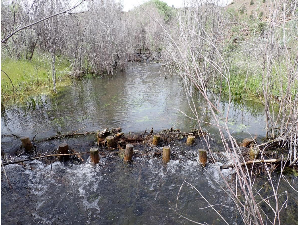
Above: View of BDA installed at a glide. Point #7
