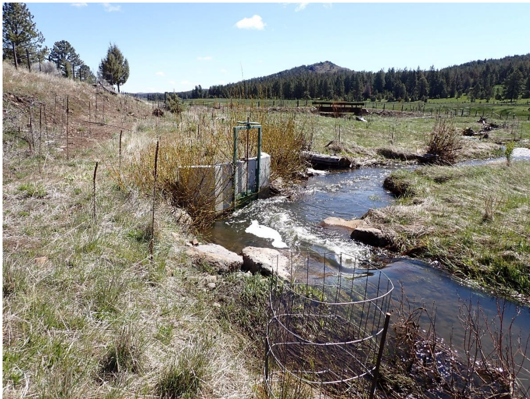
Below: Up-stream from new diversion facing west showing scour pool for efficiency.
