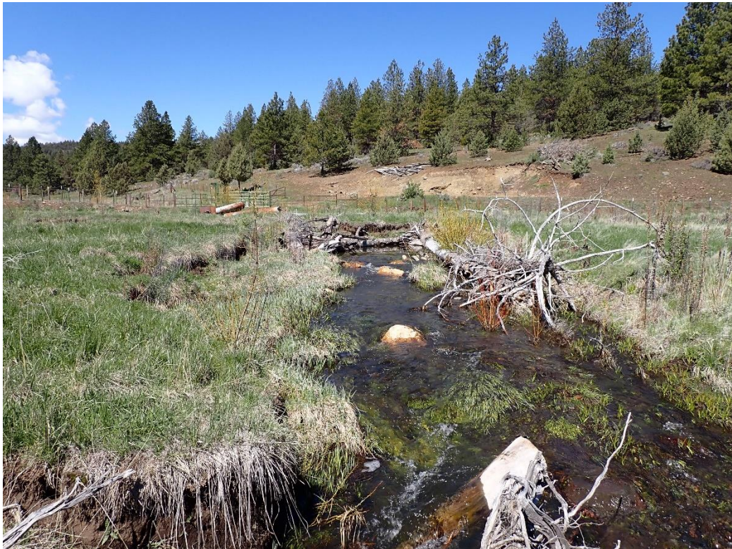
Below: Facing up-stream at in-stream work with large wood and boulder material.
