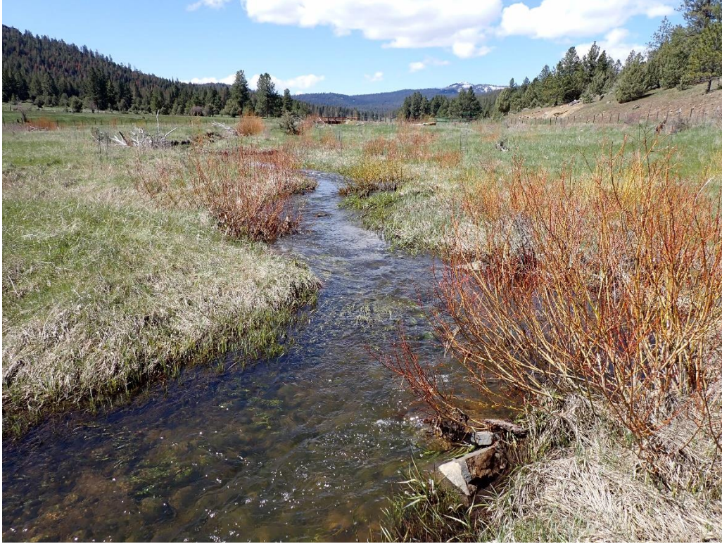
Above: Looking up-stream at in-stream work of large wood and rock materials.
